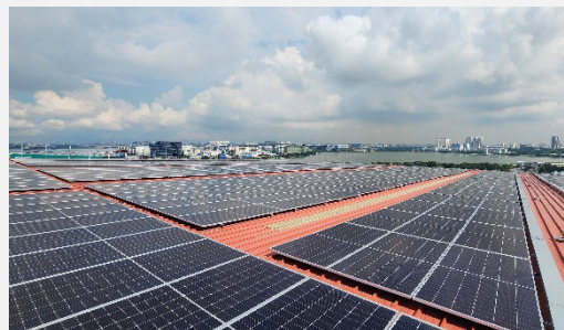
Rooftop solar panels at 4 Pandan Avenue
